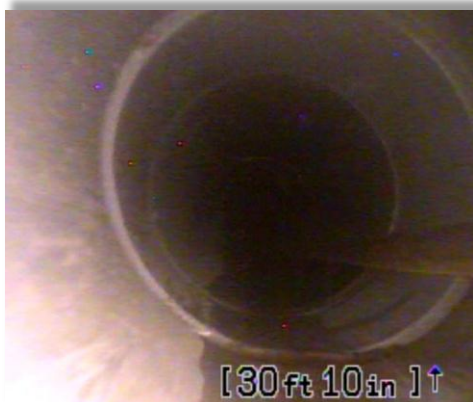
Picture of before the Flow-Liner® installation, showing water infiltrating into the bottom of the existing conduit
