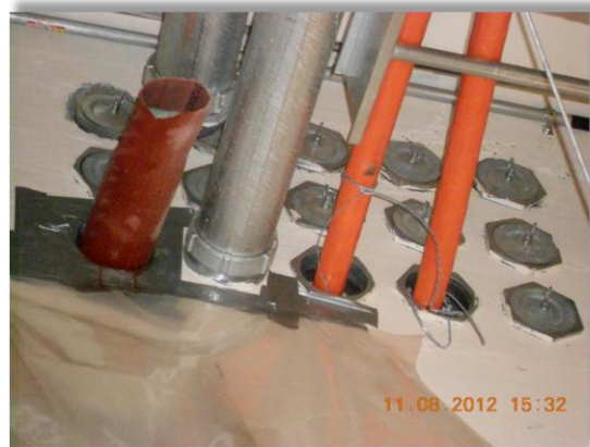
Picture of the Flow-Liner CIP Conduit® (on left) after it was inverted into the telecommunication conduit
