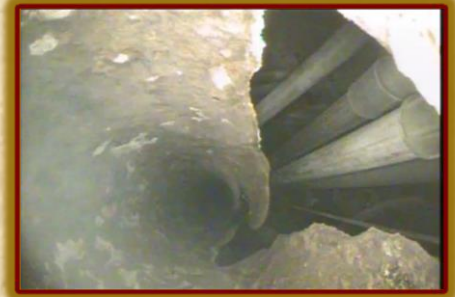
Deteriorated Cast iron pipe prior to lining
